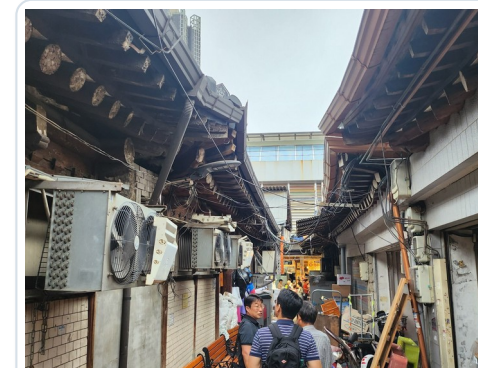
Fire-safety and access constraints
